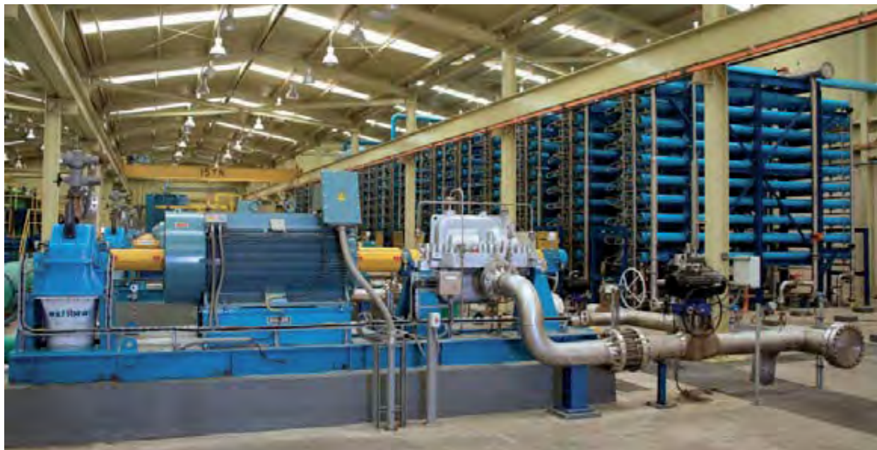
ADASA's desalination plant in the city of Antofagasta.
